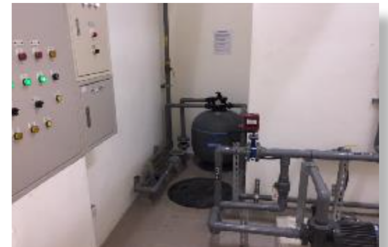
Rainwater harvesting storage system
