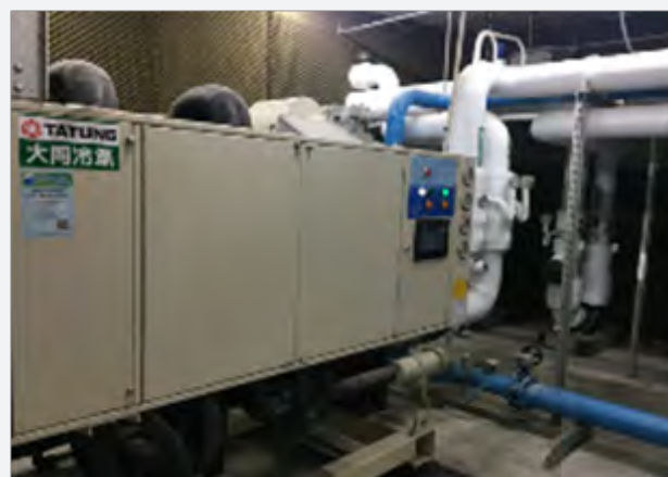
Adopting qualified machines with energy saving labels for the central air conditioning system
