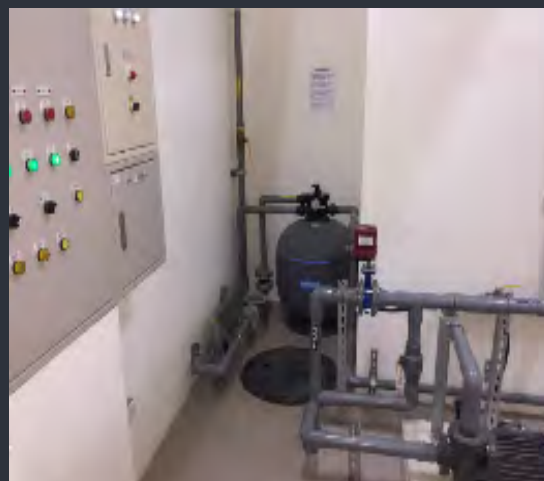
Rainwater harvesting storage system
